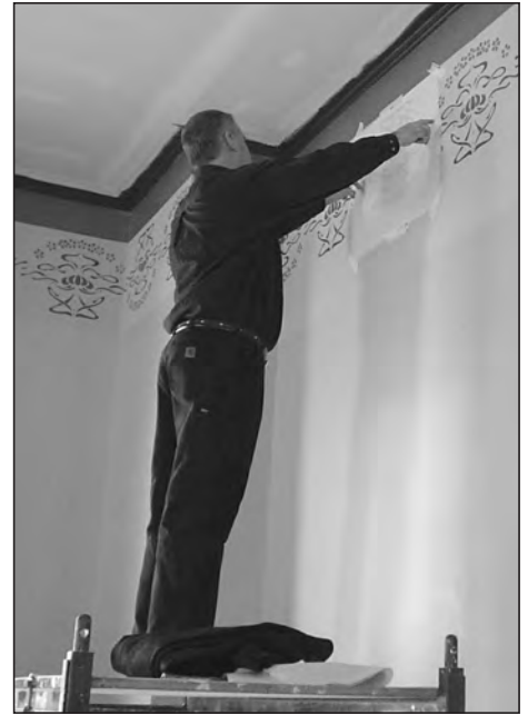
Interior specialist Alan Cloutier prepares a stencil to repair damaged stencil art in Keeney Hall.
